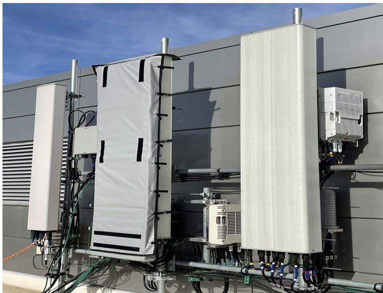
Figure 4: ConcealFab Front Absorber Kit installed on a site antenna
