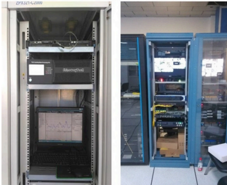
Equipment rack in monitoring centre ←
